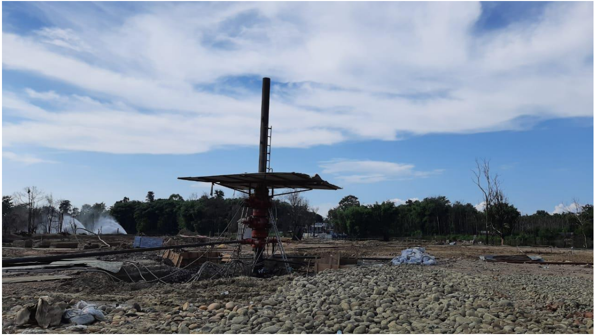
Baghjan well no 5 after diversion of flow of gas to nearby Early Production Setup (EPS)
