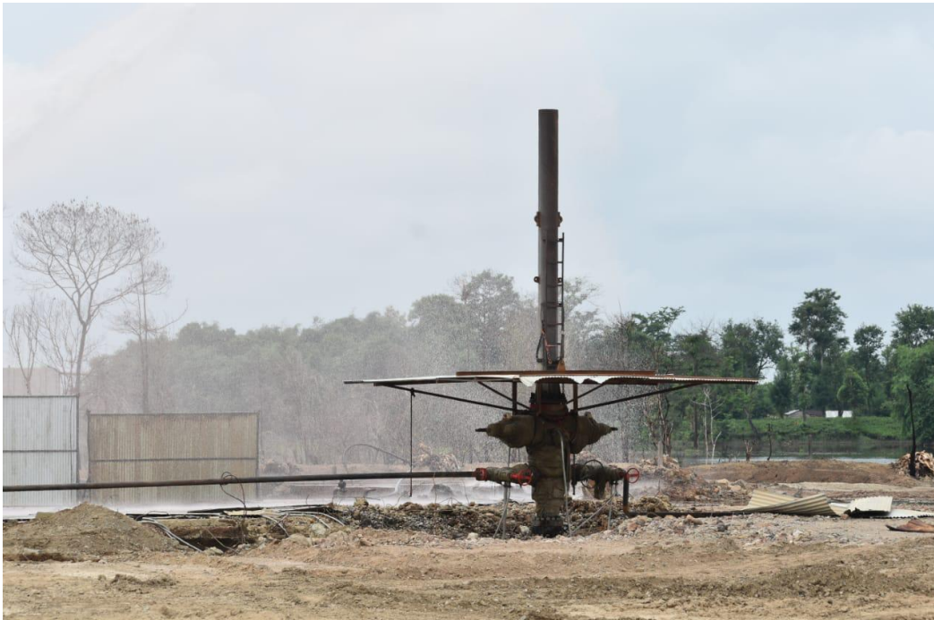
Baghjan blowout well 5 after gas diversion carried out successfully
